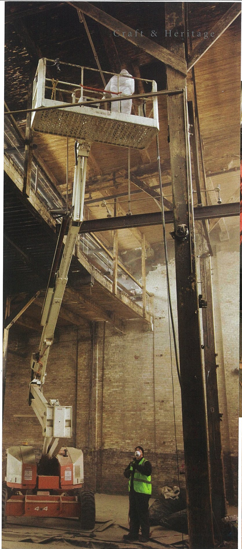
Above and opposite: An industrial heritage building adaptive reuse success: In its heyday, this Douglas fir framed Roundhouse had 32 engine repair bays covering almost 100,000 sq.ft. Today, it is the downtown showcase home of Leon's Furniture.
