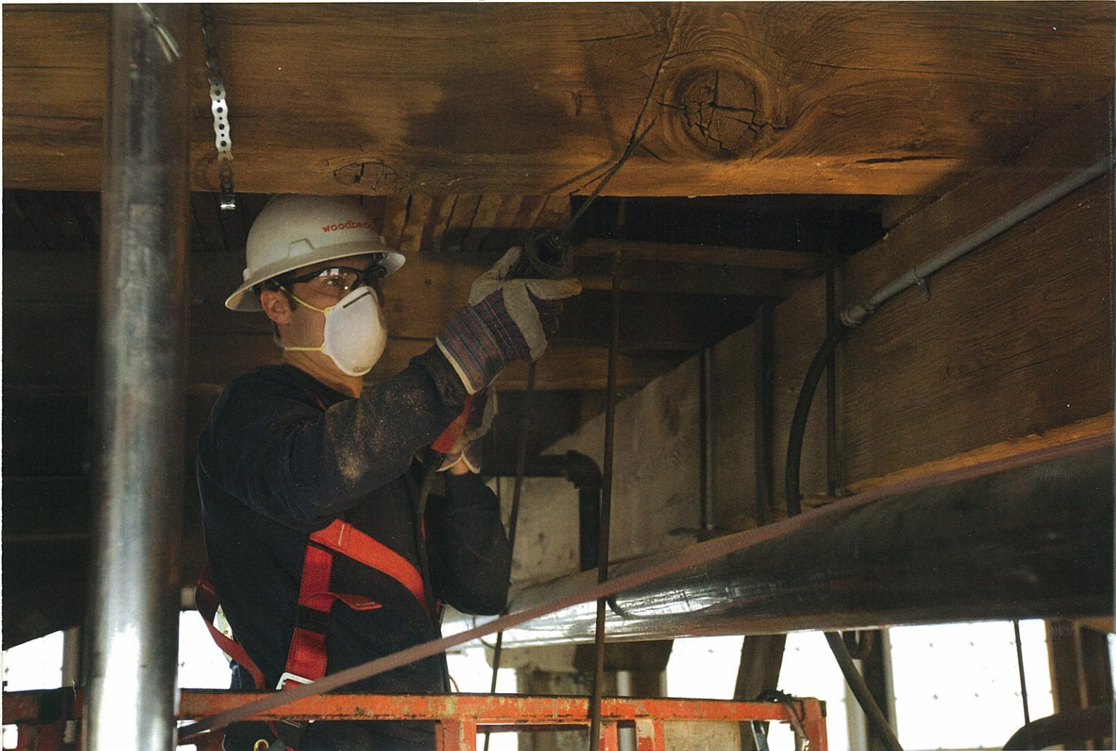
Above and opposite: The old growth Douglas fir structural frame of the Roundhouse was in remarkably good condition. A series of strap braces were installed where timbers had begun to split and twist; and missing pieces of cross bracing, railings and walkways were matched and replaced with new or recycled timber pieces sourced from across Canada.
